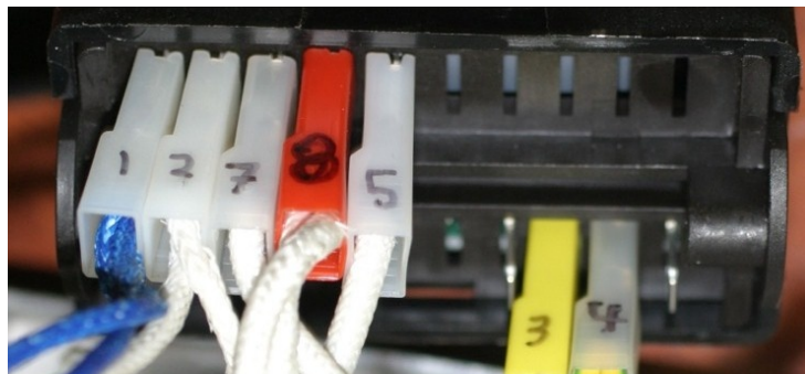
Below: Note the empty terminals on the new board (left of 3 and right of 4)
